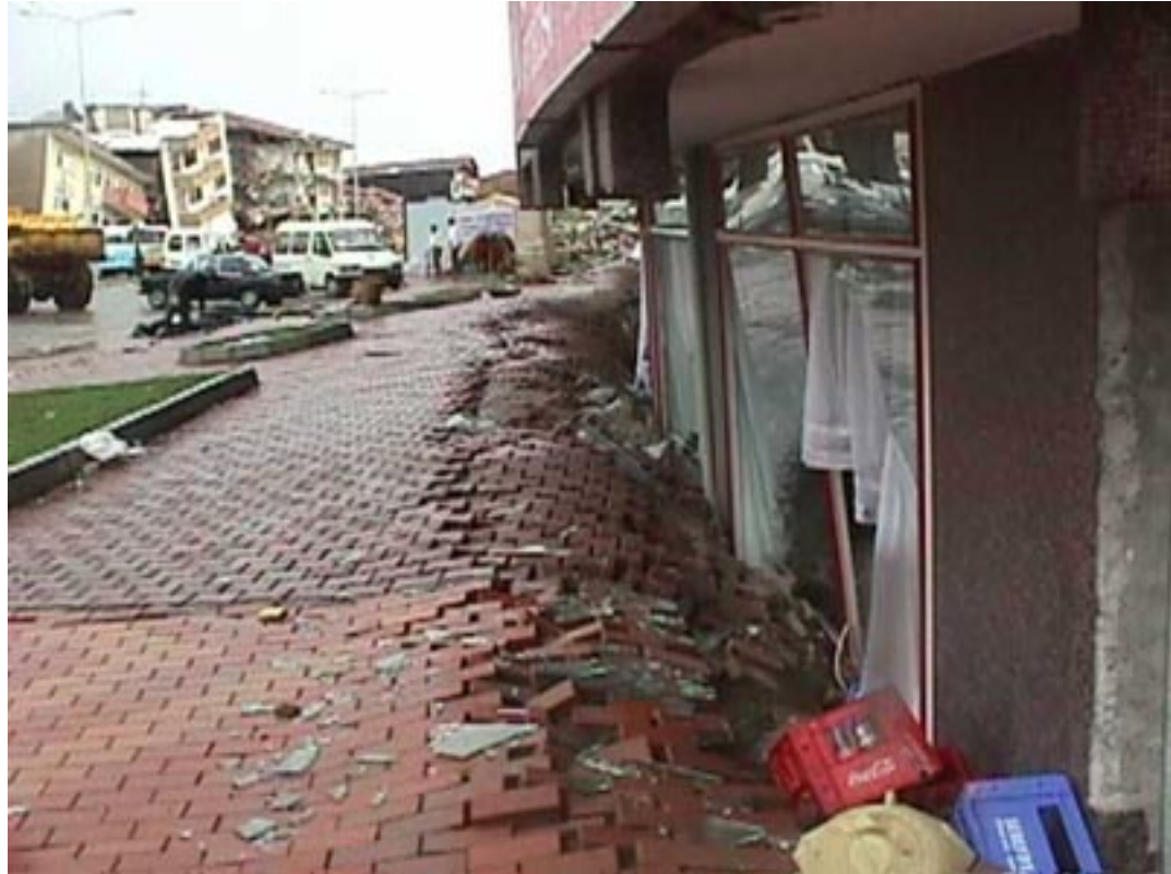
M7.6 earthquake Izmit, Turkey, 1999
